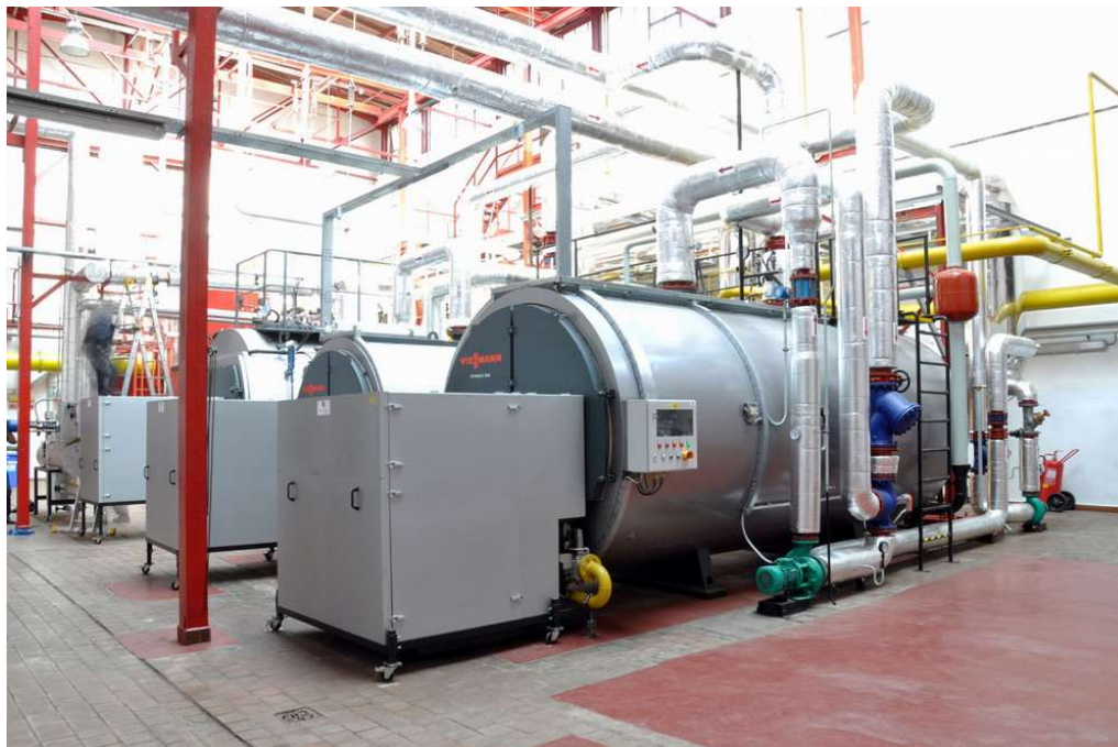
Obr. 25: Kotelna Thomayerova nemocnice [7]
