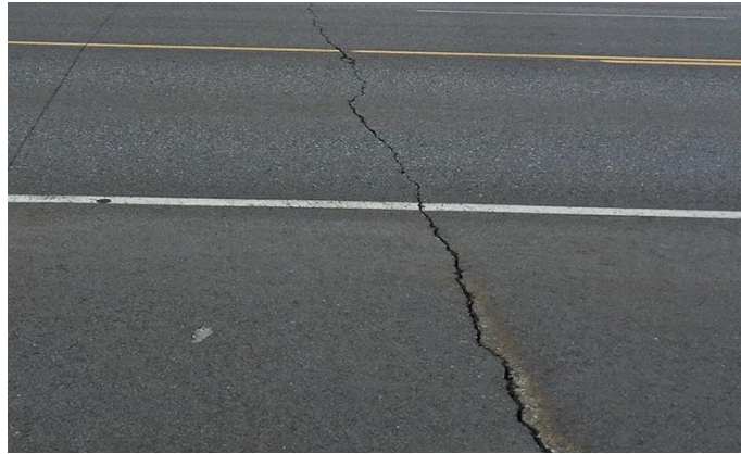
Figure 2.16 Thermal cracking of the asphalt pavement [76]
