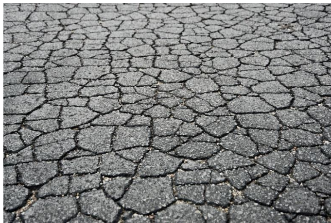
Figure 2.15 Fatigue (crocodile/alligator) cracking of the asphalt pavement [74]
