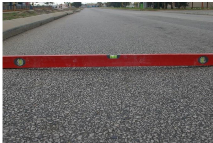
Figure 2.14 Rutting of the asphalt pavement, adapted from [72]
