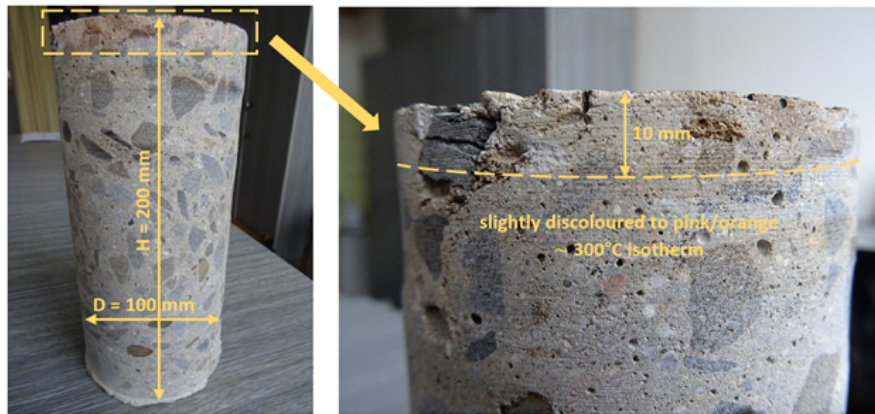
Figure 22: Concrete core “WA.2” – estimation of approximate damage depth using colorimetry method.
