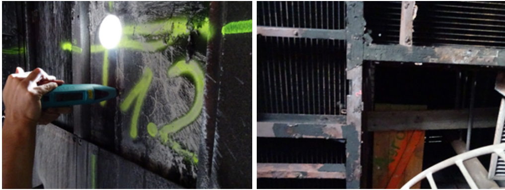
Figure 18: Left: conducting rebound hammer test; right: steel specimen cut out of floor beam in “ZONE 2”.
