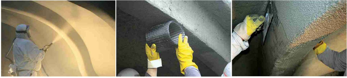
Figure 2-12: Application of TRC reinforcing layer on a historic roof structure in Zwickau, Germany [Sch09]
