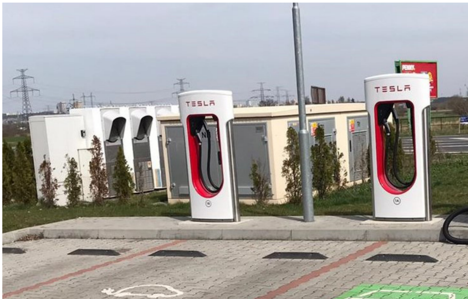
Tesla Supercharger - stojan s kabelama
