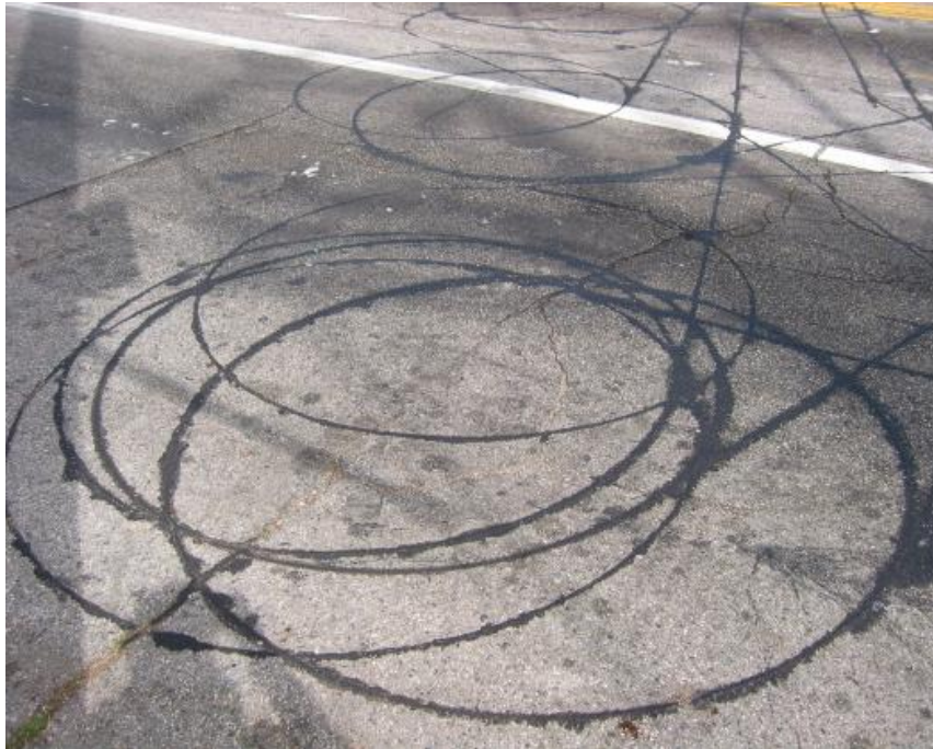
Figure 7: Close-up look of old and new induction loops cut in the pavement (17)
