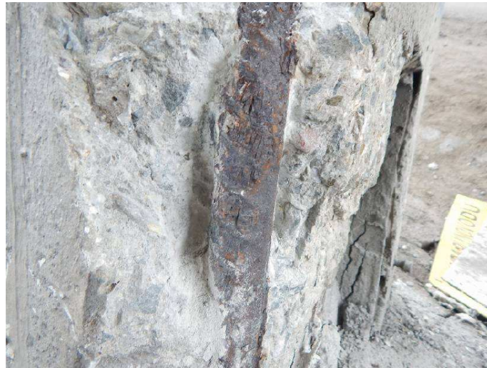
Figure 4.11: Investigation of reinforcement corrosion at the strut with spalled concrete cover [46]
