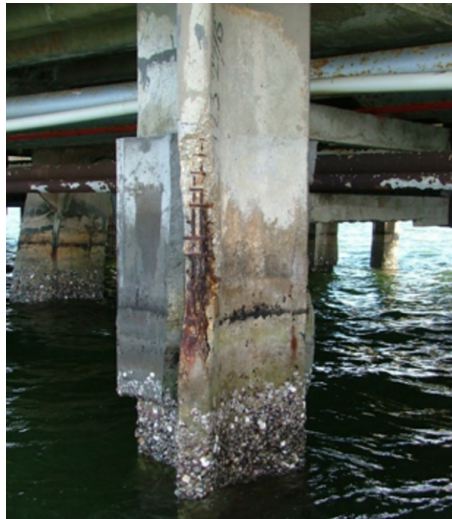
Figure 2.15: Corrosion of reinforcement attacked by sea water [117]
