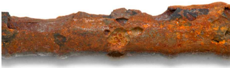
Figure 2.5: Steel rebar corroded due to chloride ingress [67]
