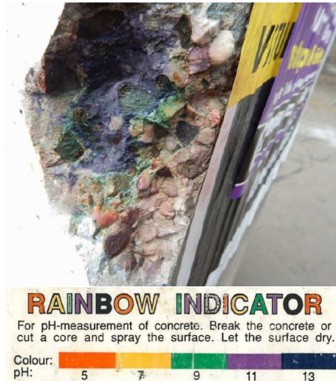
Figure 4.3: Characteristic evolution of carbonation, test site P1 with measured carbonation depth 20 mm. Rainbow indicator 0-15 mm with pH 5, 15-20 mm with pH 9 and >20 mm with pH 11-13 [46]
