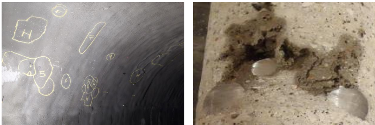
Fig. 46 Hollow spots identified by hammer tapping (left), core showing poor embedment of steel bars (right)
