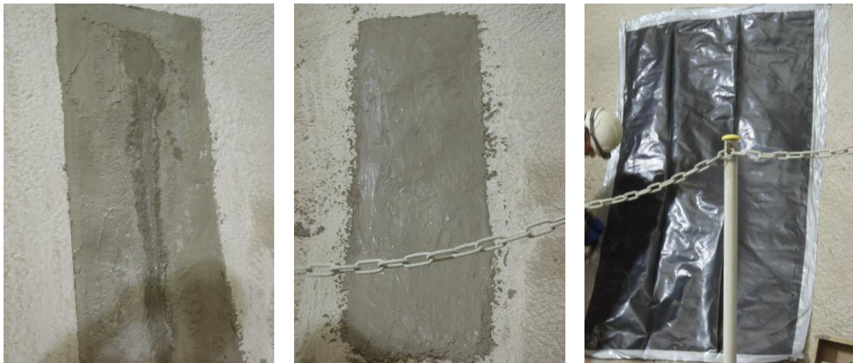
Fig. 57 Application of fast setting mortar – water ingress (left), water ingress sealed (middle) and curing protection (right)
