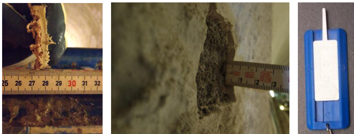
Fig. 51 Dry patch thickness (left and middle) and depth gauge for wet thickness test (right)
