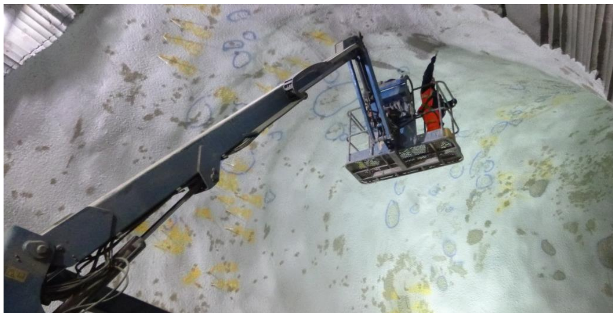
Fig. 62 Visual inspection of pin holes
