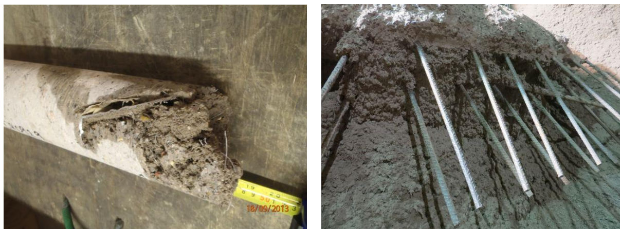
Fig. 41 Quality issues with continuity bars
