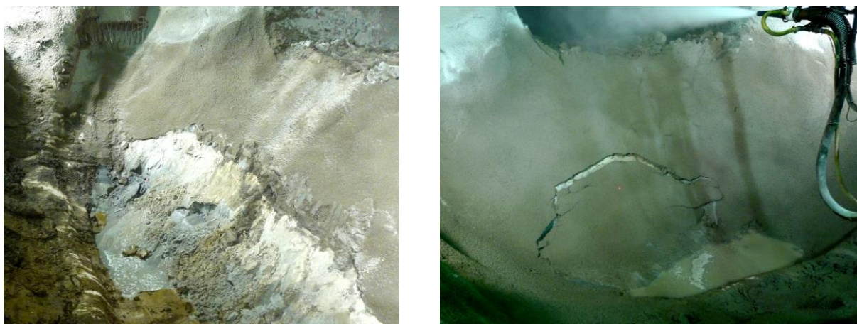
Fig. 26 Tunnel face with flowing sand (left) difficult to be sealed with shotcrete (right)
