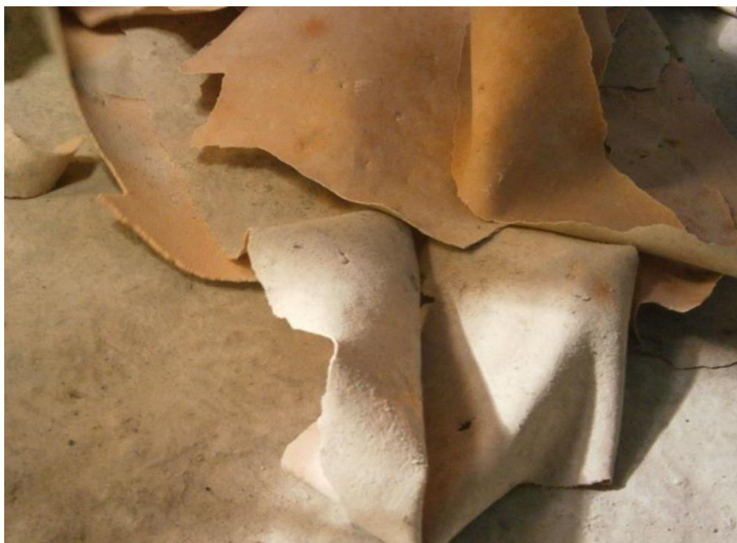
Fig. 31 Debonded spray-applied waterproofing membrane, [46]
