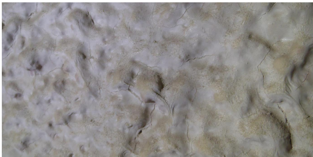
Fig. 63 Micro-cracks on the membrane's surface
