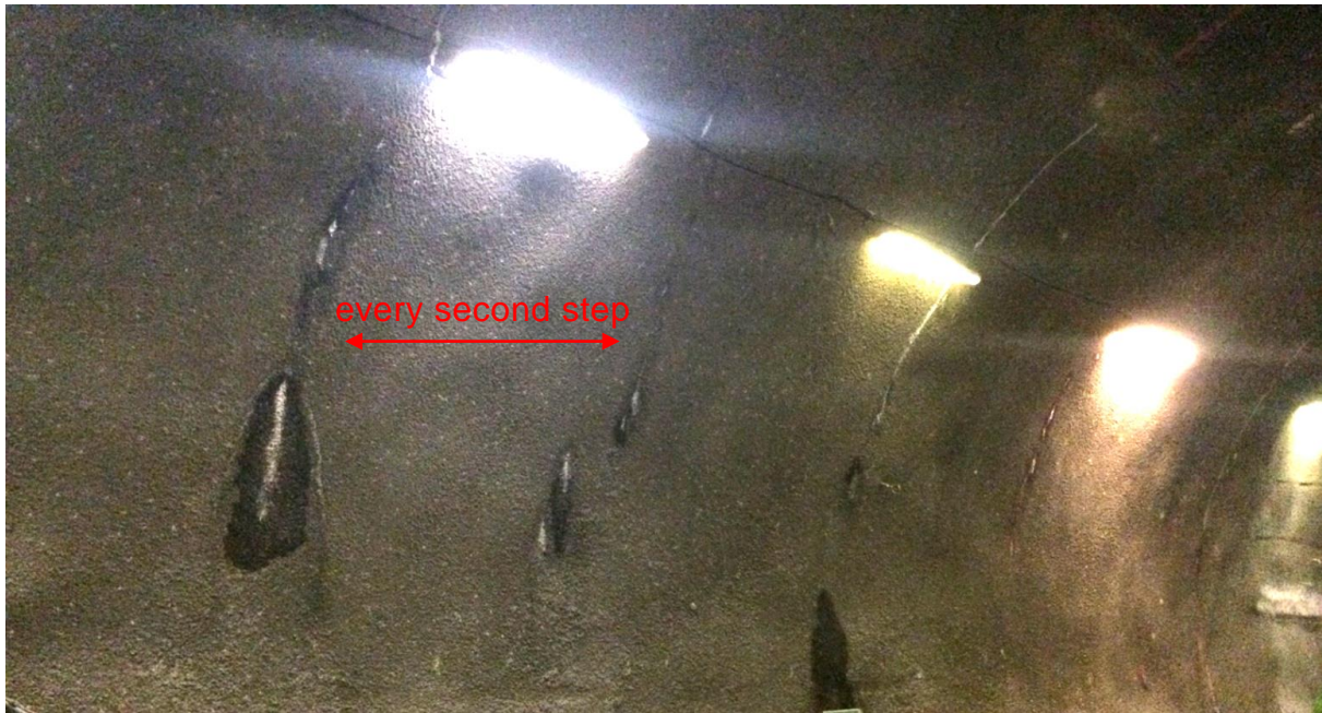
Fig. 37 Water ingress through the second layer of the primary lining
