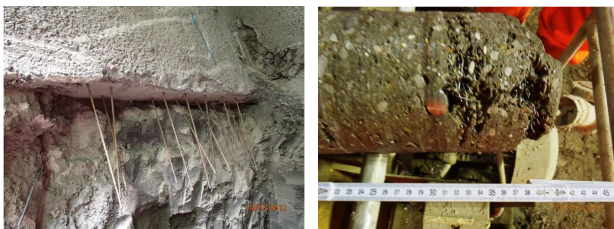
Fig. 42 Poor compaction caused by combination of steel fibres and steel bars
