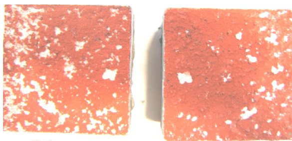
Fig. 82 Failure in cohesion of coloured EVA-based spray-applied waterproofing membrane, [13]
