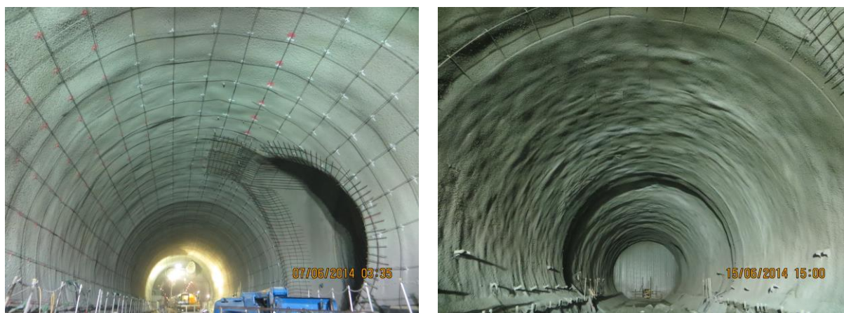
Fig. 65 Guidance profile bars (left), final layer of sprayed concrete secondary lining (right)
