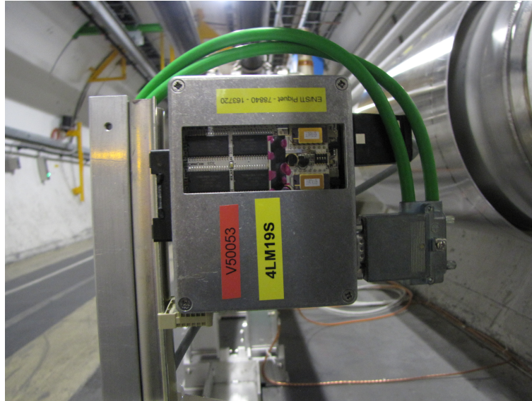
Figure 1.2: A RadMon installed in the LHC. The serial number V50053 , and device ID 4LM19S can be seen. Note the heavy fieldbus cables (green). Image from [3].
