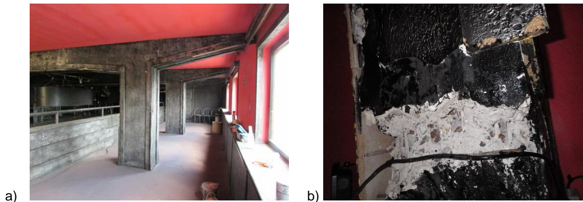
Figure 3.9: a) 3NP transverse beams at column line A looking south b) Damage at 2015 probe location (Beam at Level 3NP, Column Line 5)
