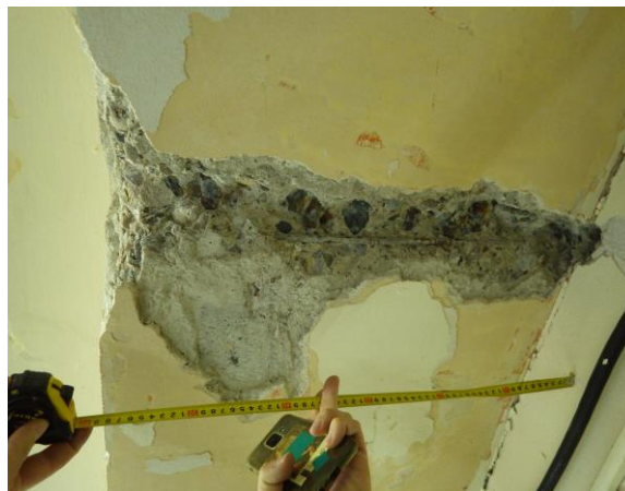
Figure 3.11: Longitudinal Beam Damage from 2015 at Level 2NP, Column Line A, Between 8 and 9
