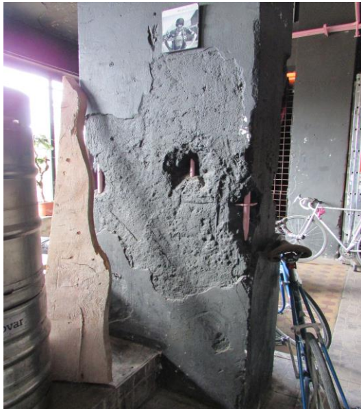
Figure 3.7: Column damage from 2015 above Level 1PP at column lines A-4
