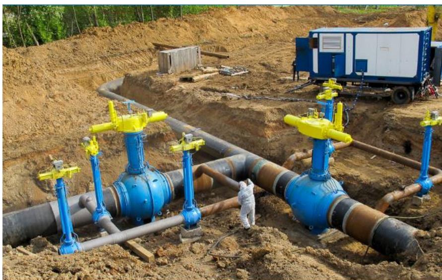
Figure 4 - Block valve station [35]
