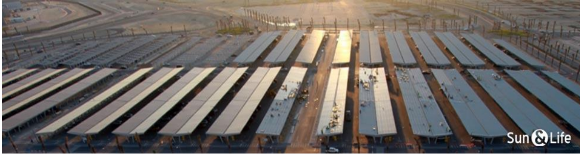
Figure 3.7: The 10 MW Photovoltaic Carport System in Saudi Arabia [7]
