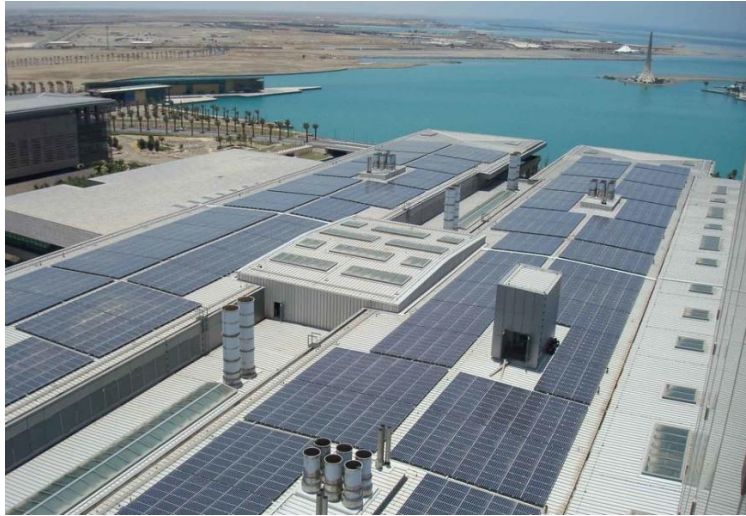
Figure 3.5: The 2 MW rooftop solar plant at KAUST [7]
