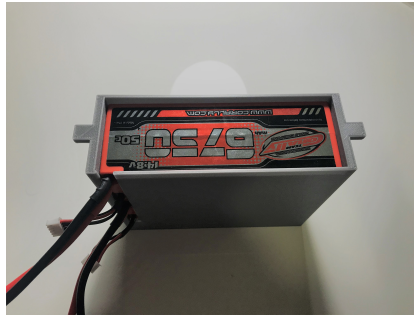
(b) : Batteries in the battery box
