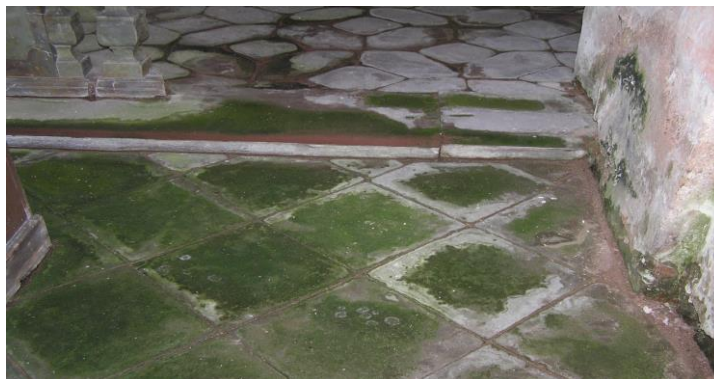
Picture 35: Moisture, biological degradation - internal wall and floor (St. Anna's Church)
