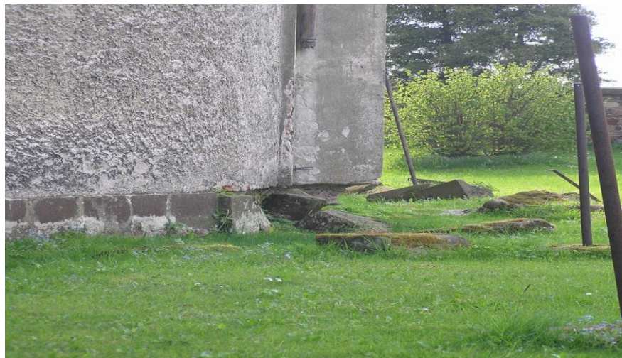
Picture 23: Deterioration of the external wall
