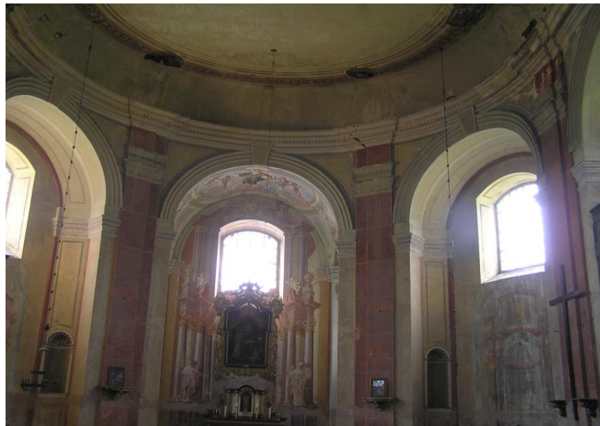
Picture 29, 30: Cracks of the internal wall and ceiling (St. Anna's Church)
