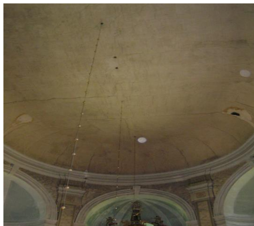
Picutre 28: Cracks of the Ceiling ( St. Barbara's Church)
