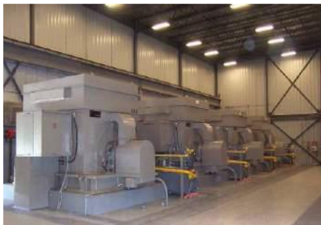
Fig. 3. Granite Substation Condenser Hall [20].
