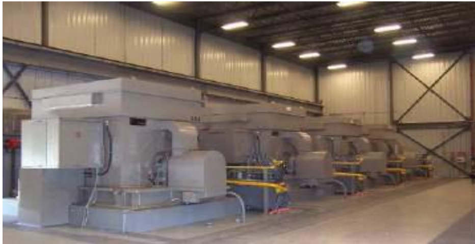
Fig. 3.10: Granite substation condenser hall [180].
