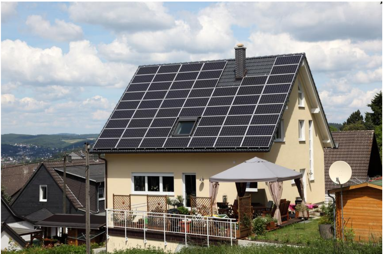
Fig. 27 Example of rooftop PV installation [27]
