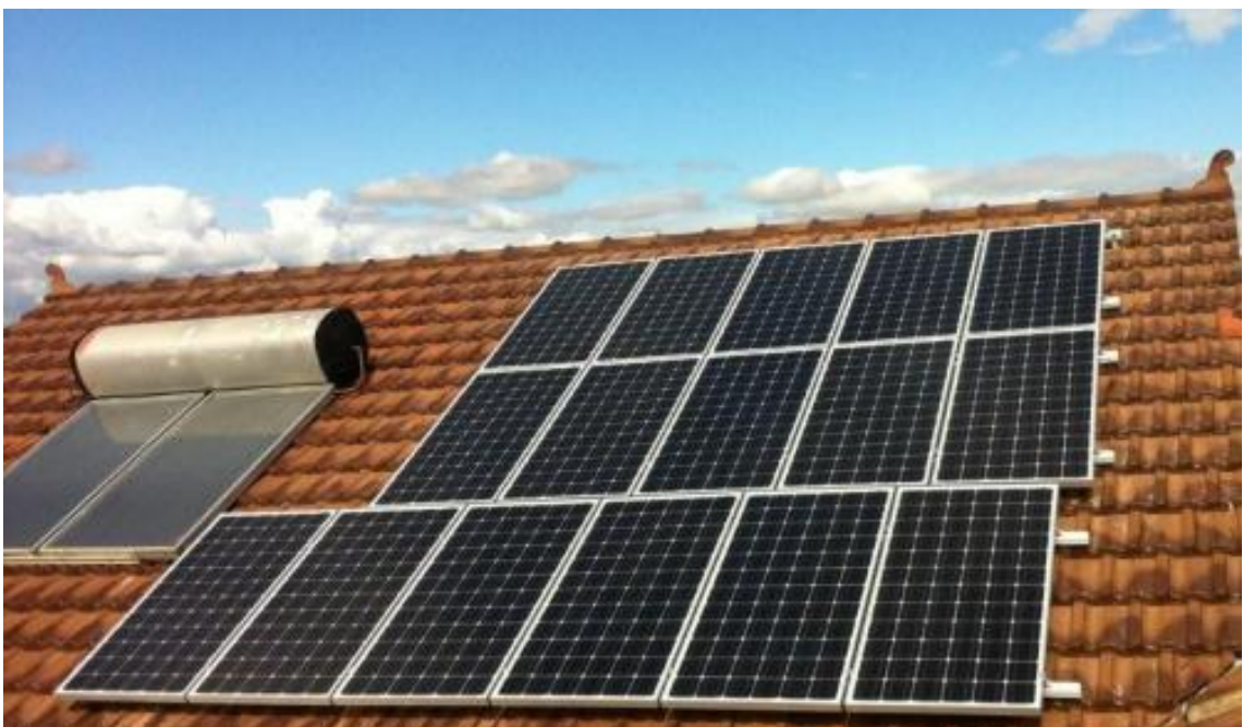
Fig.44 Ordinary rooftop Solar system [43]
