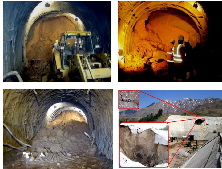
FIGURE 4. The development of the collapse and slope failure.
