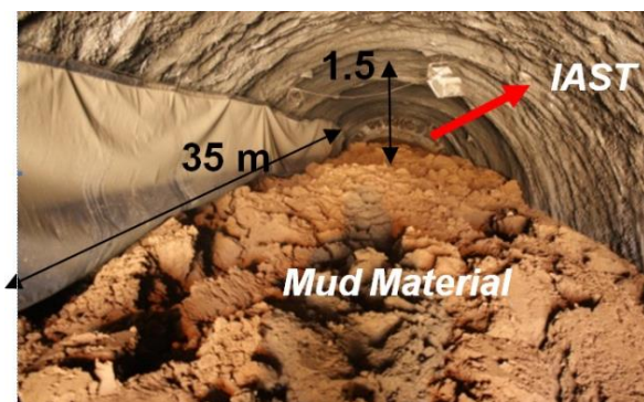
FIGURE 11. The mud flow running into the tunnel.
