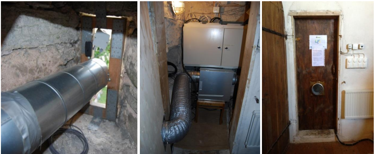
Figure 5.13 Left - the air intake and outdoor sensor. Middle - the fan and the flexible air duct. Right - the new temporary tower door.
