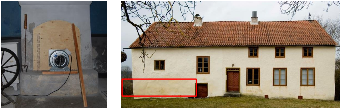
Figure 5.5 Left - the exhaust fan mounted in a wooden board used for sealing. Right - the investigation was carried out in the bottom floor of the left (southern) lower part of the split-levelled building.
