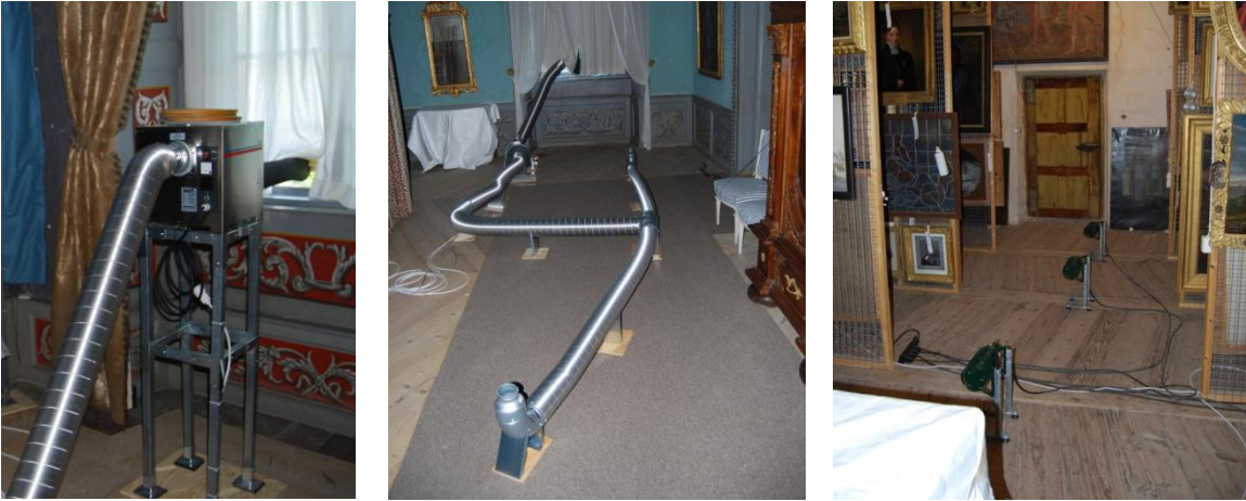
Figure 6.10 Left, dehumidifier in the room “Grå rummet”. Middle, adaptive ventilation in the room “Blå rummet”. Right, conservation heating in the room “London”.
