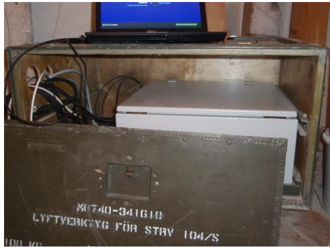
Figure 5.2 The cabinet with control equipment.
