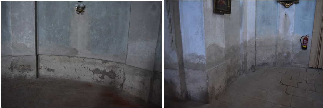
Figure 4.14. Discoloration due to previous interventions and humidity level
