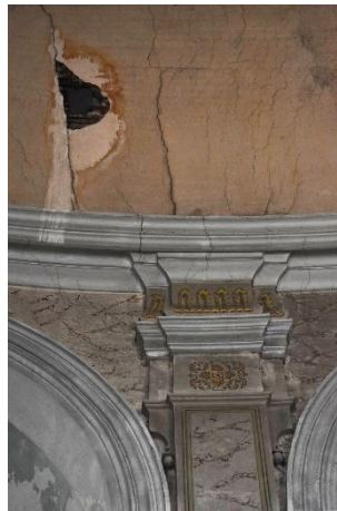
Figure 4.13. Cracks above pillar due to the concentration of stress
