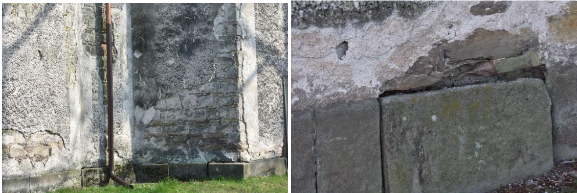
Figure 4.3. Cracks due to soil settlements
