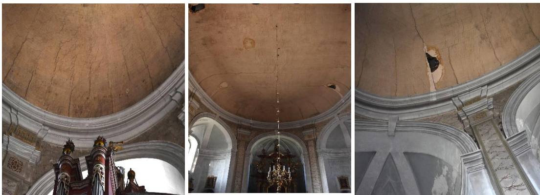
Figure 4.10. Cracks in the ceiling
