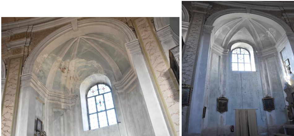
Figure 4.15. Humidity stains on the plaster
