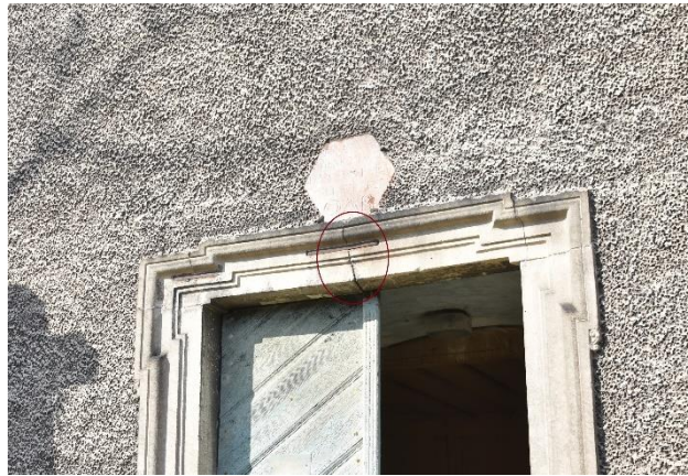
Figure 4.2. Crack in the lintel
