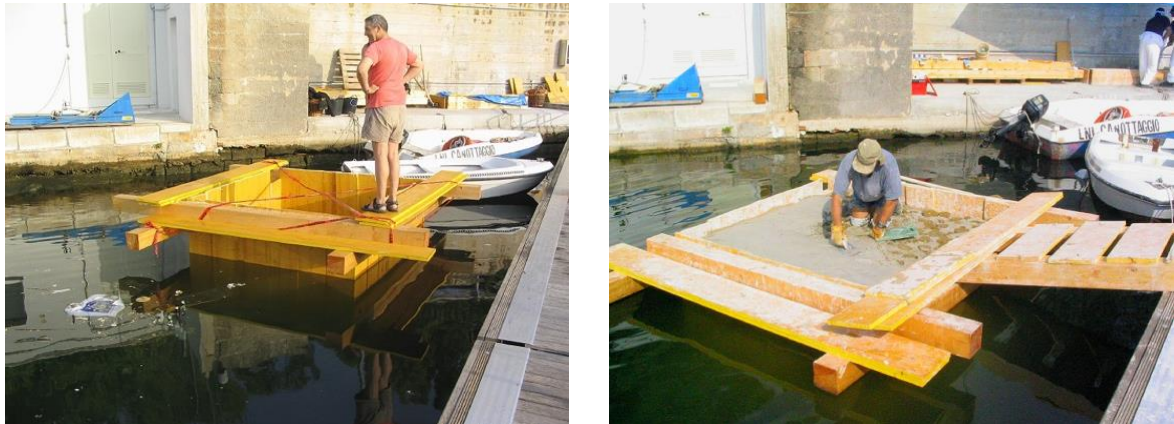
Figure 8. (left) Prepared formwork for the Brindisi pila ; (right) detailing the top surface. (J. P. Oleson et al., 2006)
