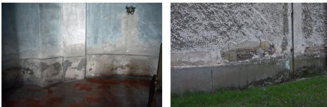
Figure 4.4: Effects of moisture and rising dampness in the church
