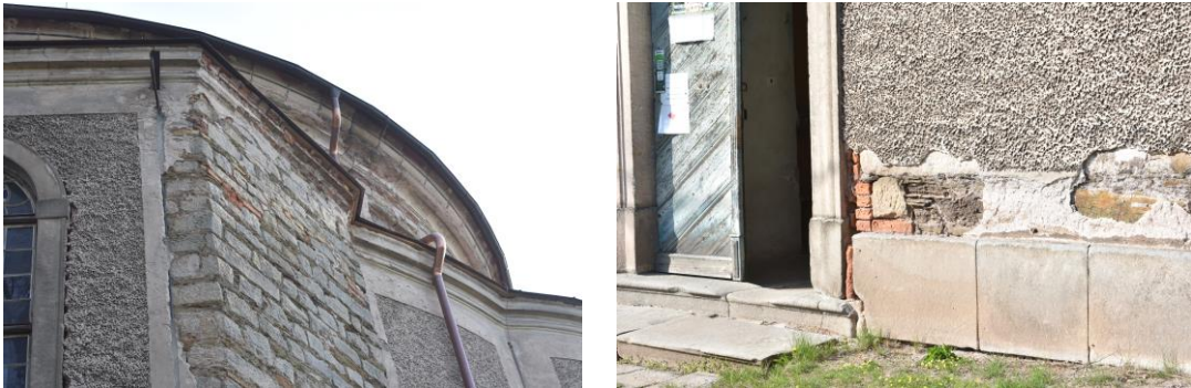
Figure 4.5: Detachment and loss of material
