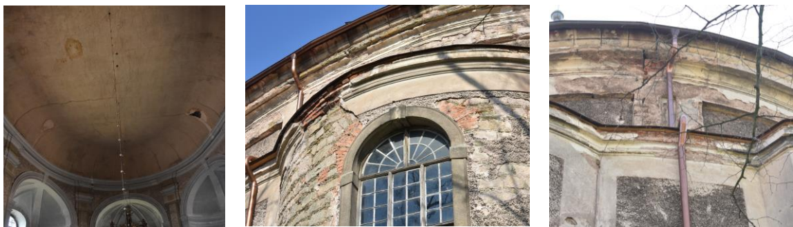
Figure 4.1 Cracks in the internal (a) and external (b) (c) walls of the church
