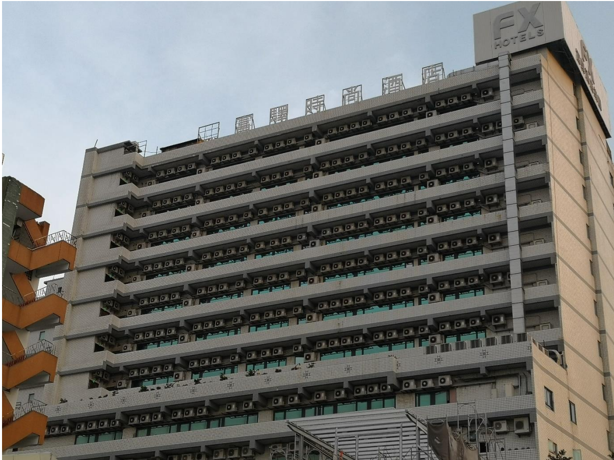
Pic. 18: AC outdoor units. FX Hotel in Tainan, Taiwan
