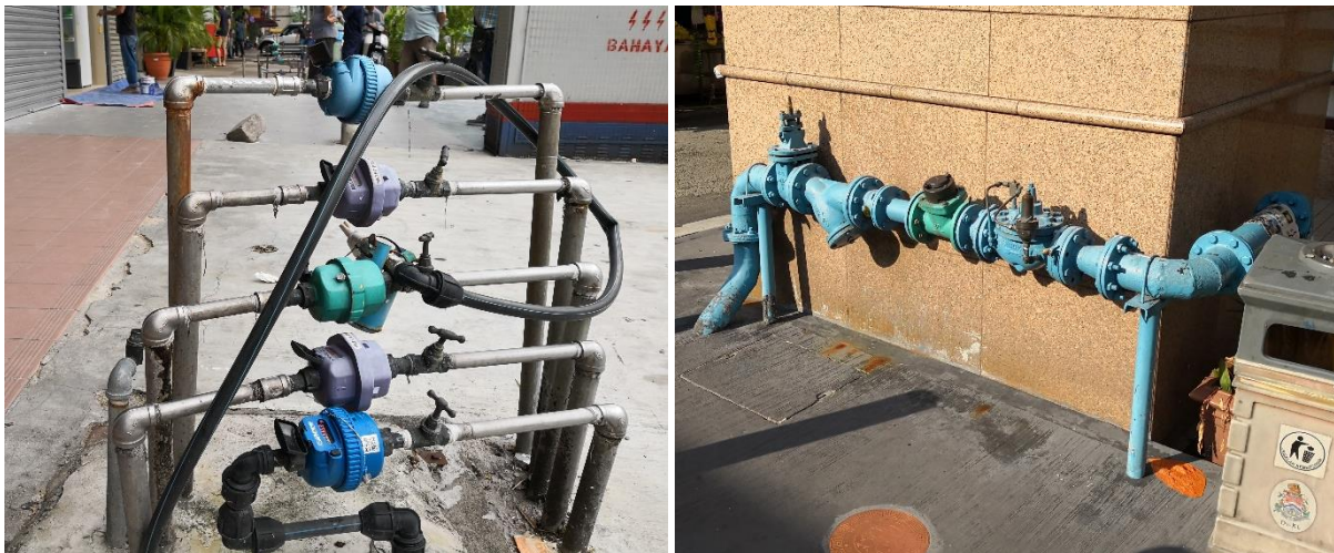
Pic. 23: Water meters (on the left) and water meter station (on the right), Kuala Lumpur, Malaysia
