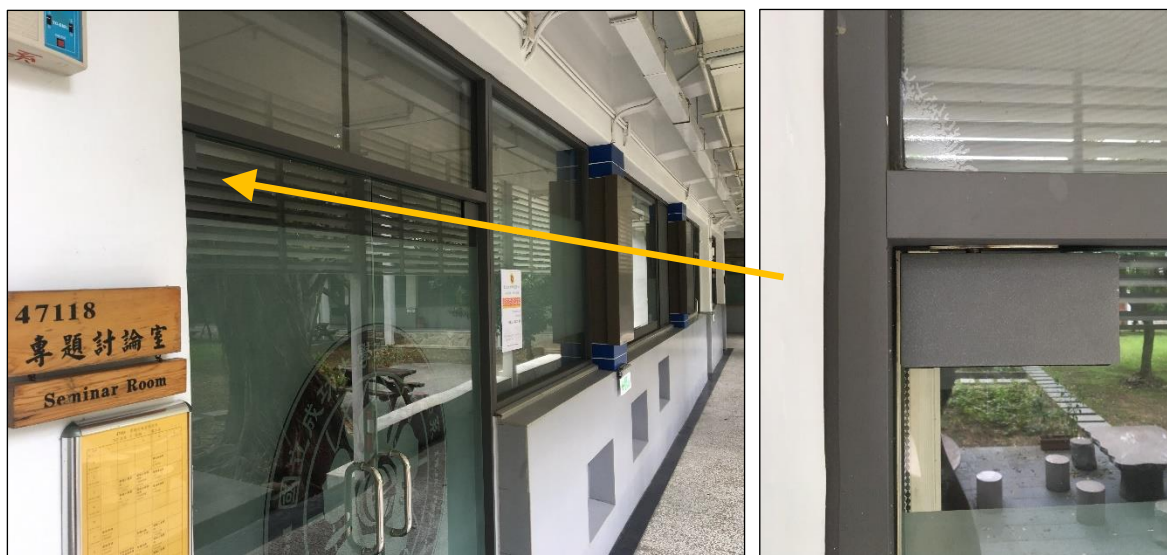
Pic. 14: An example of none airtightness construction, NCKU campus, Tainan, Taiwan
