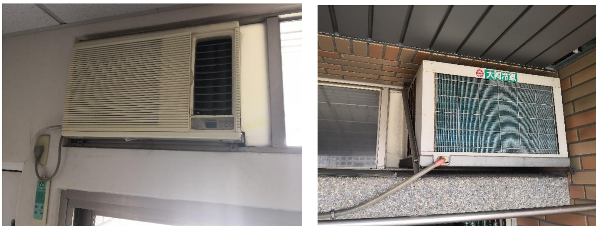
Pic. 17: Single air conditioning unit from interior (on the left), exterior (on the right). NCKU dormitory – student room, Tainan, Taiwan
