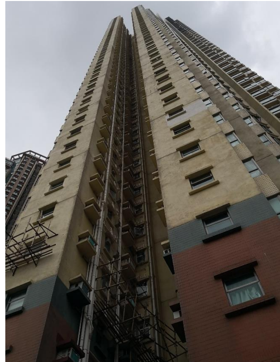
Pic. 24: Sewerage along the facade, residential building, Singapore
