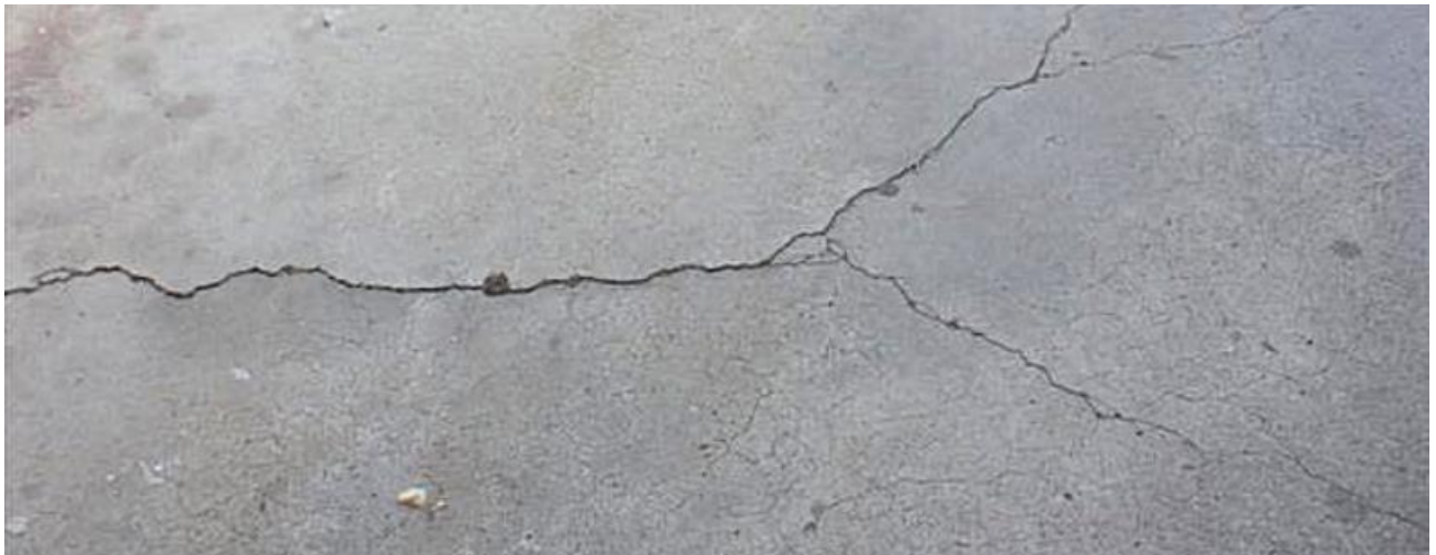
Fig. 2.2.1.1 Picture of cracks, caused by plastic shrinkage
