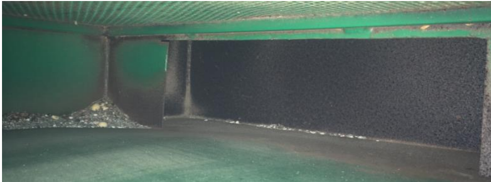
Figure 25. Dust and contaminating particles accumulation.
