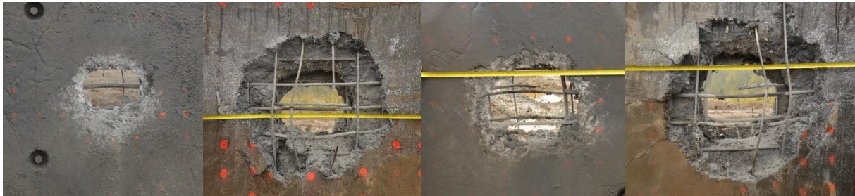
Figure 10 Specimen No. 21 after contact blast loading, 2.8 kg charge left left contact side, left right soffit, 4.2 kg charge right left contact side, right right soffit
