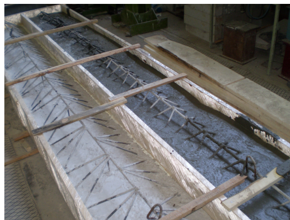
FIGURE 4. The look of sandwich reinforced concrete-foamed concrete floor slabs during concrete casting by foamed concrete or foamed concrete with fibre polypropylene.
