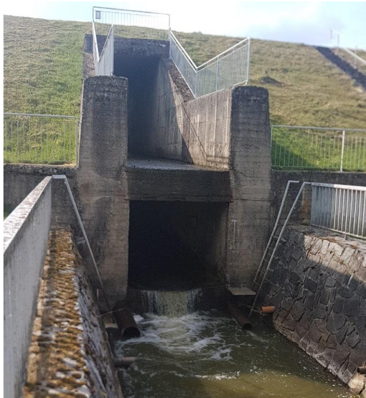
Figure 32 - The spillway chute (up), the tailrace (down) and a part of the stilling basin [30]
