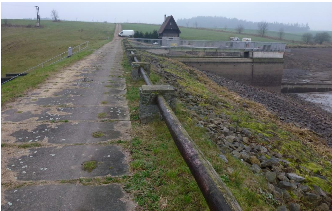
Figure 28 - The crest of the dam and the upstream slope with the multipurpose control structure [28]
