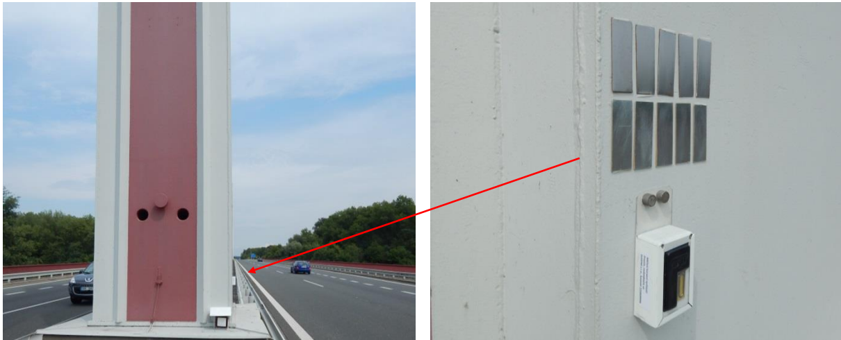
Fig. 16. Example of flat coupons and Fe-AirCorr sensor on highway bridge.
