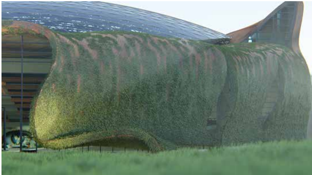
EXTERNAL WALLS view looking at the weathered and foliage covered facade
