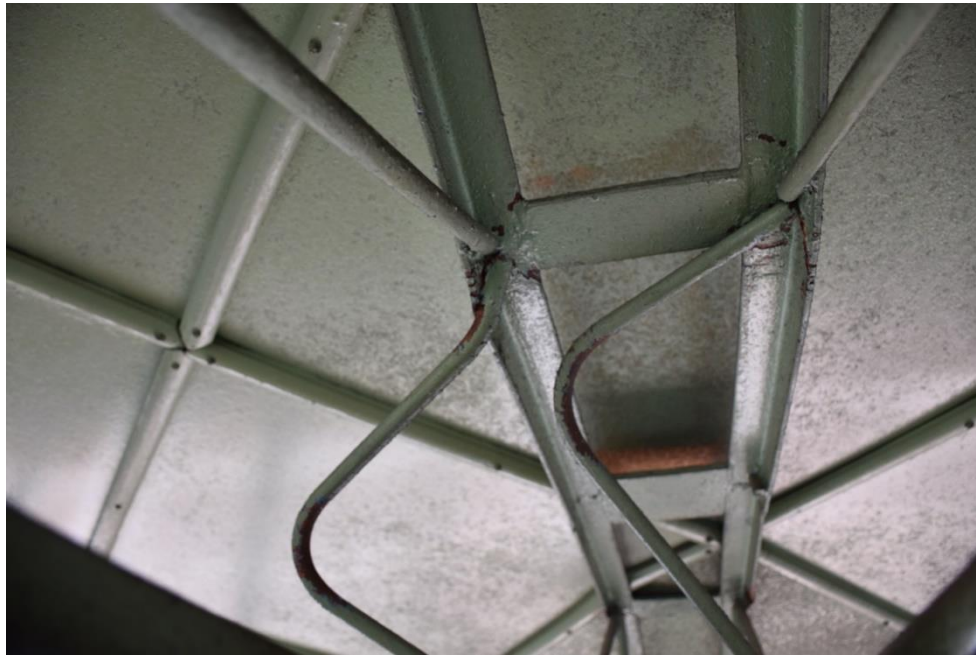
Figure 2.10 Buckling of diagonals
