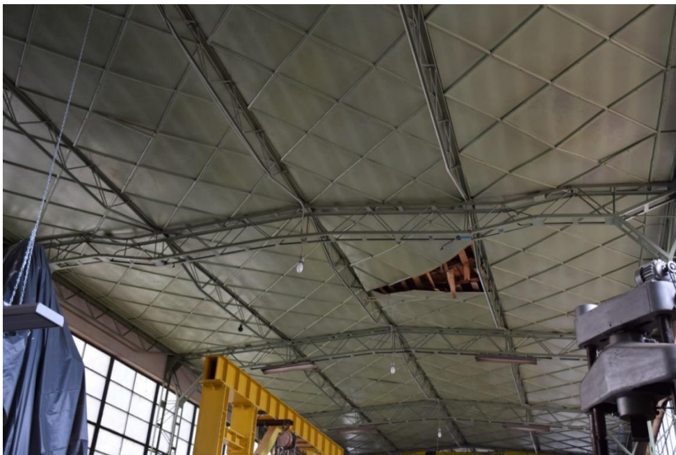
Figure 2.7 The girder from the frame in axis 4 after the storm
