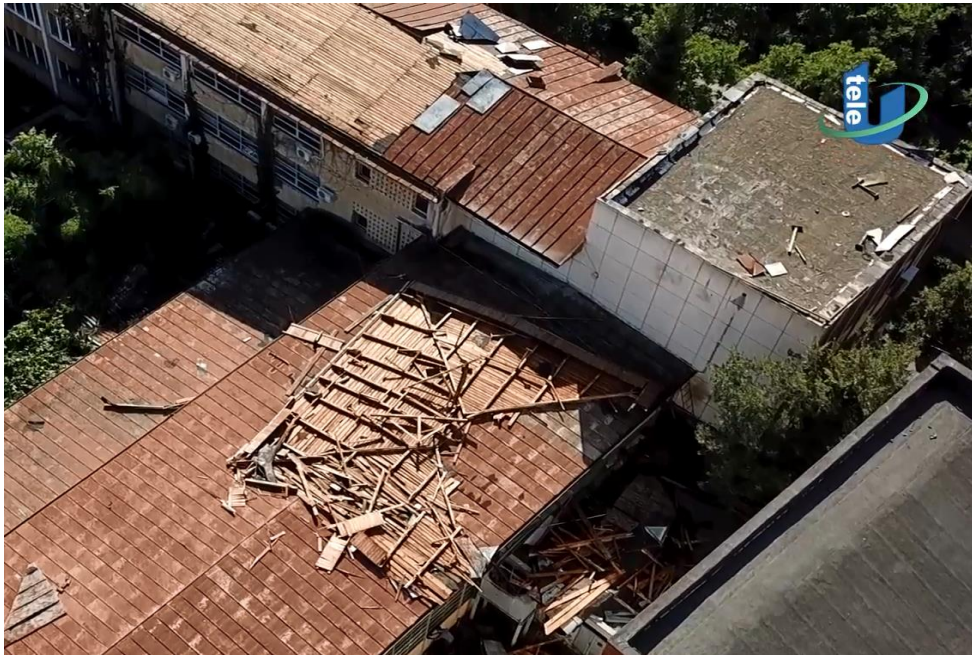
Figure 2.6 Top view of the hall after the storm
