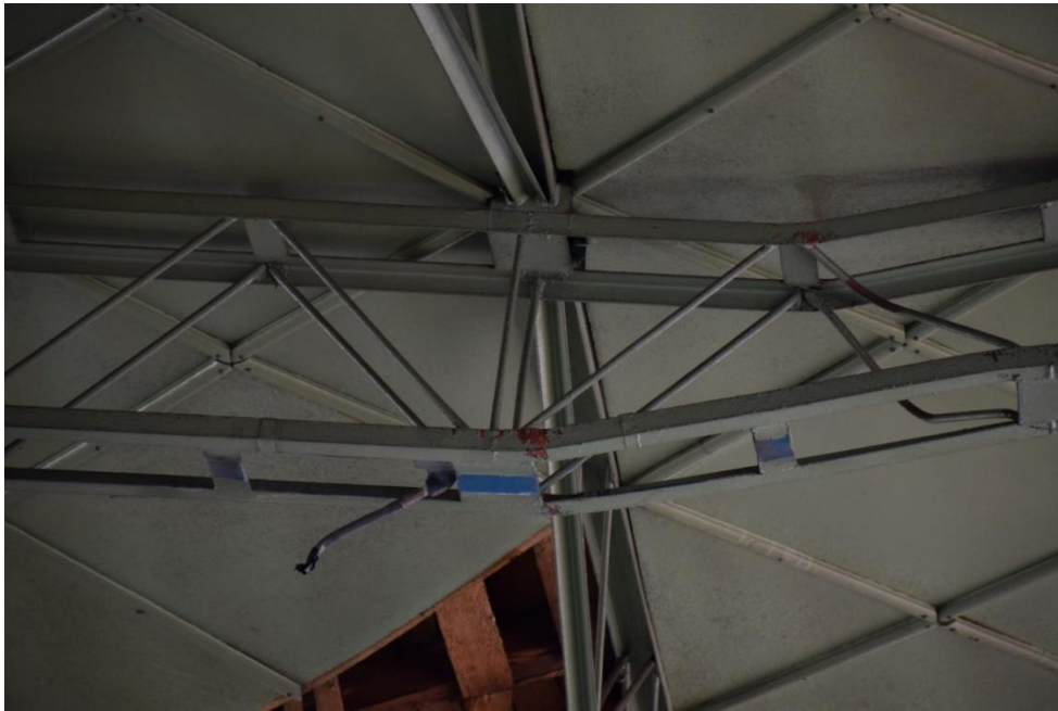
Figure 2.8 Deformation of the girder angles and buckling of diagonals
