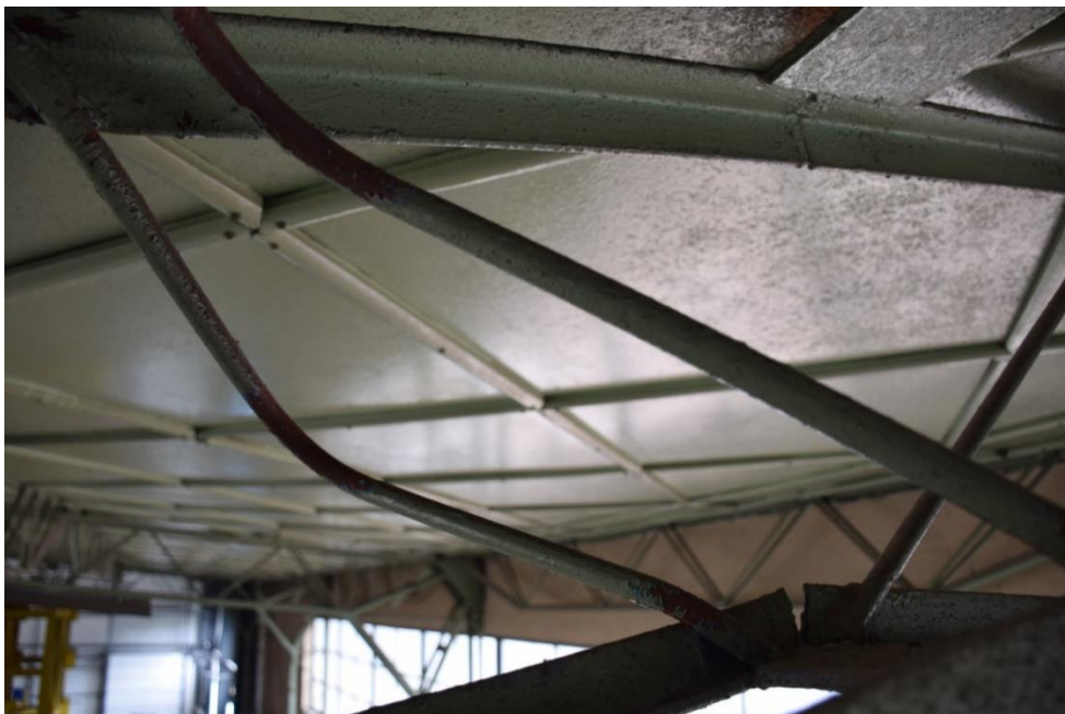
Figure 2.9 Cracking of the continuity weld of the angles
