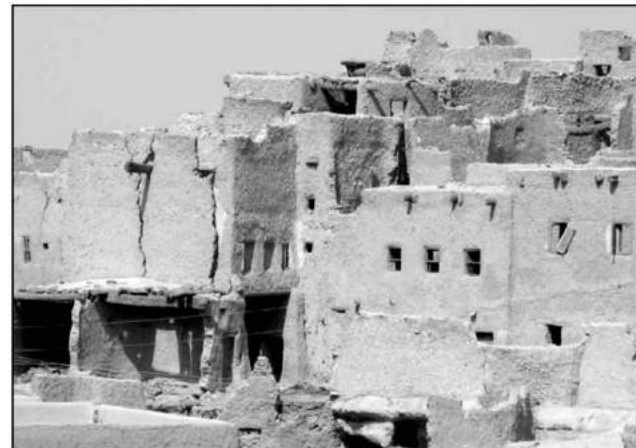
Fractures under the palm beams in the walls.
