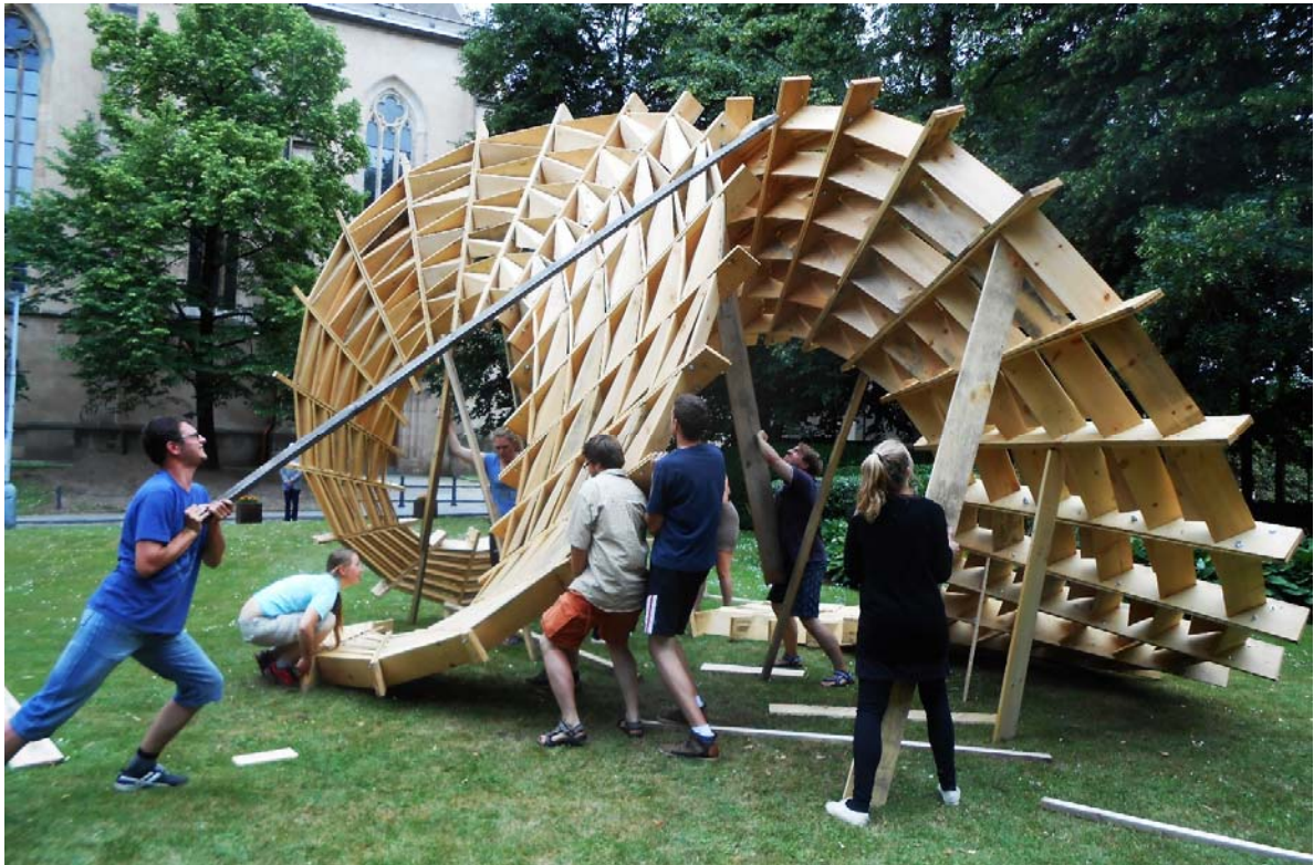
Figure 6: LOOP Pavilion Building (photo: Davidová 2014)
