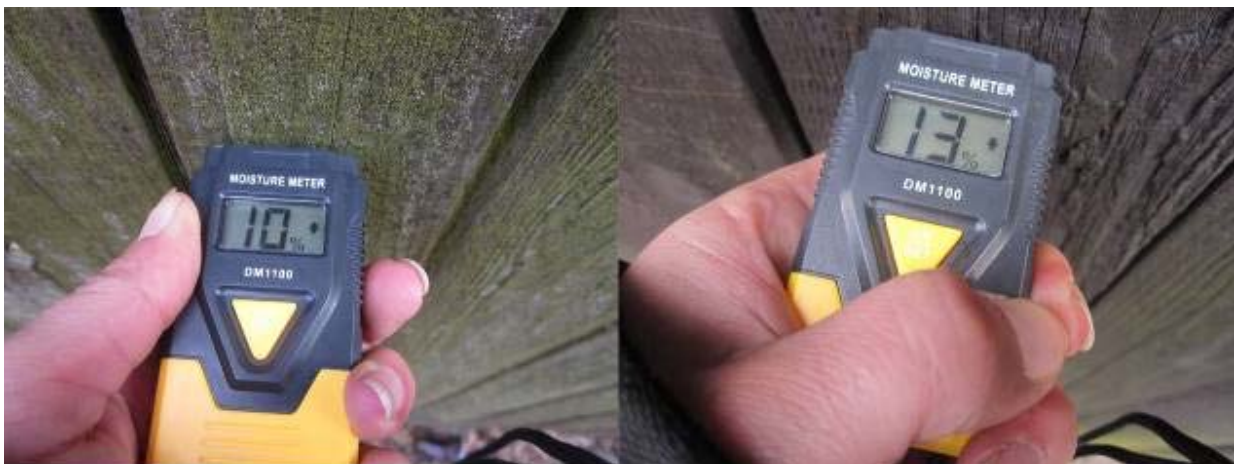
Figure 15: Fence with and without Algae Measured with Moisture Meter, Nové Město nad Metují (photo: Davidová 2013)
