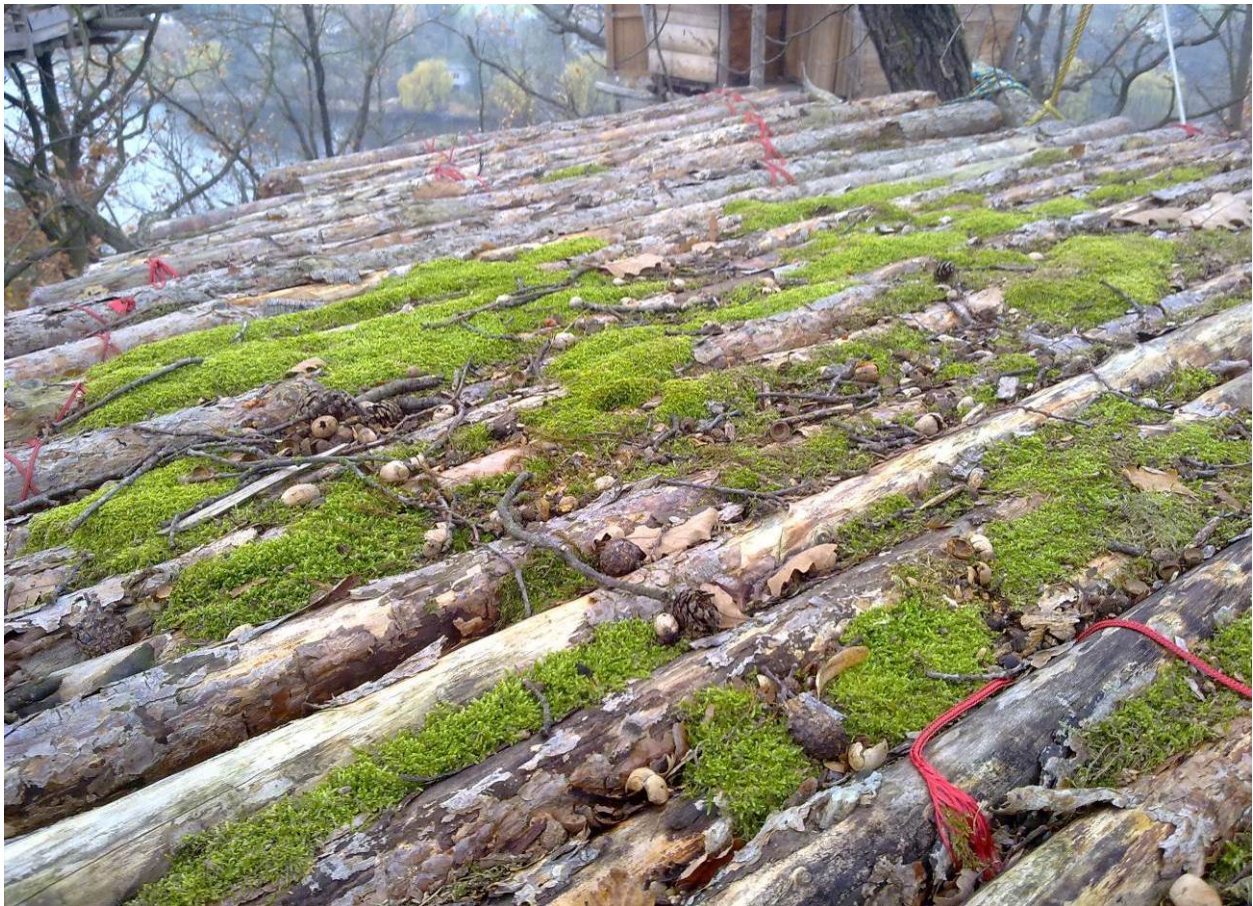
Figure 46: Davidová & Závada: SpiralTreeHouse - Local Moss Inhabiting the Platform after One Year of Seeding. Notice the Habitation Based on the Structural Direction of the Logs (photo: Davidová 2012)
