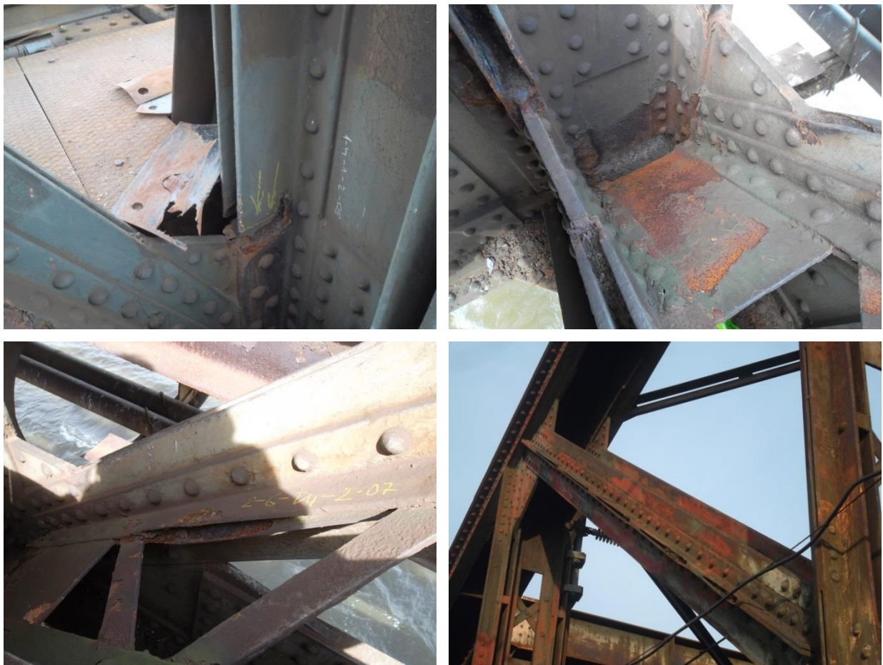
Figure 17 - Deterioration on the bridge. A, B (top) reduction of section in the connection elements. C,D (bottom) deformation on angles.
