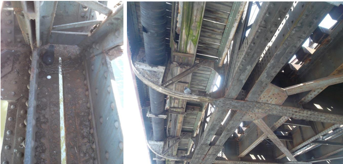
Figure 18. Biological sources of decay on the bridge.
