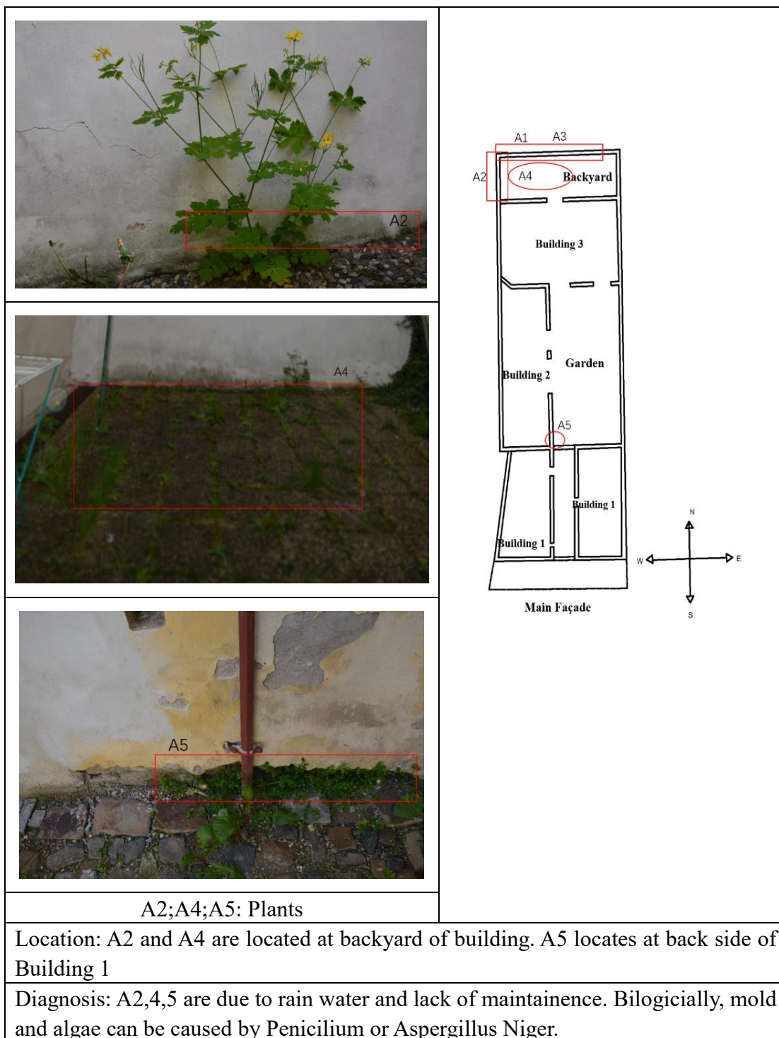
Figure 16: Bio-deterioration by Plants
