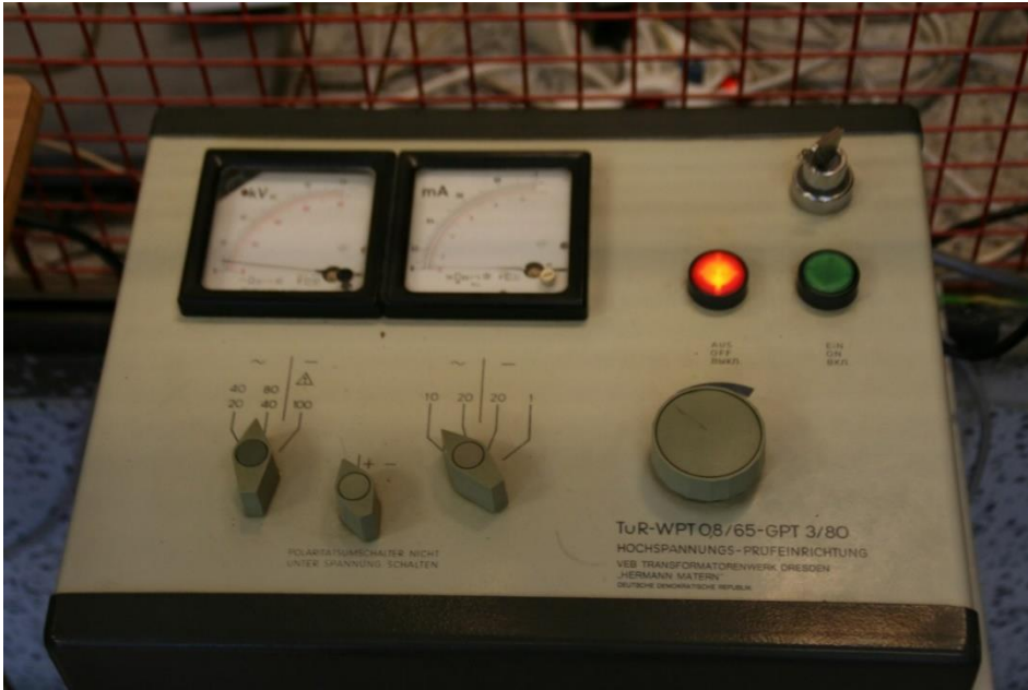
Figure 9 – AC power supply control station
