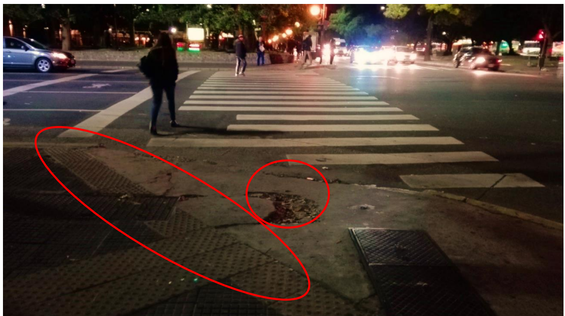
Fig. 24: Damaged access to a pedestrian crossing and incorrectly used tactile ground surface indicators
