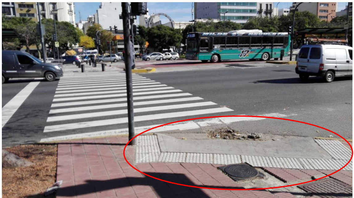
Fig. 30: Damaged dropped curb with wrong usage of tactile paving, Back edge is missing
