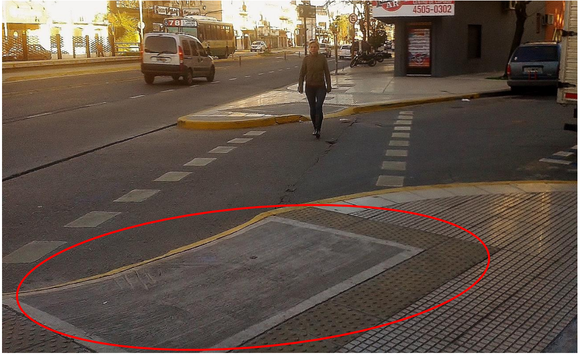
Fig. 38: Incorrectly installed dropped curb with tactile paving
