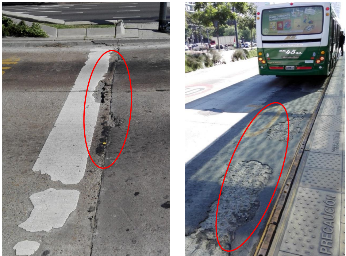
Fig. 29: Some signs of wear and potholes on the busway
