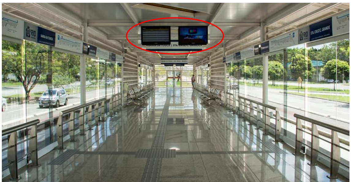
Fig. 53: Inside the station, at the top of the picture there is static and real-time passenger information (54)
