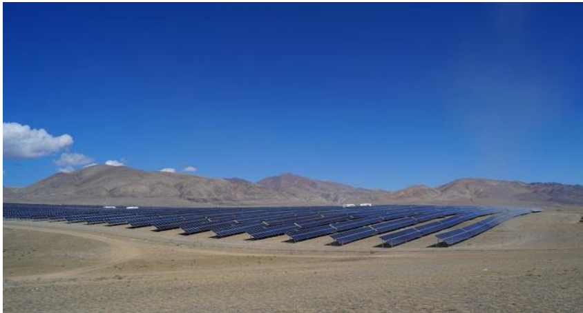
Figure 14 – Solar Power Plant using PV – system.
