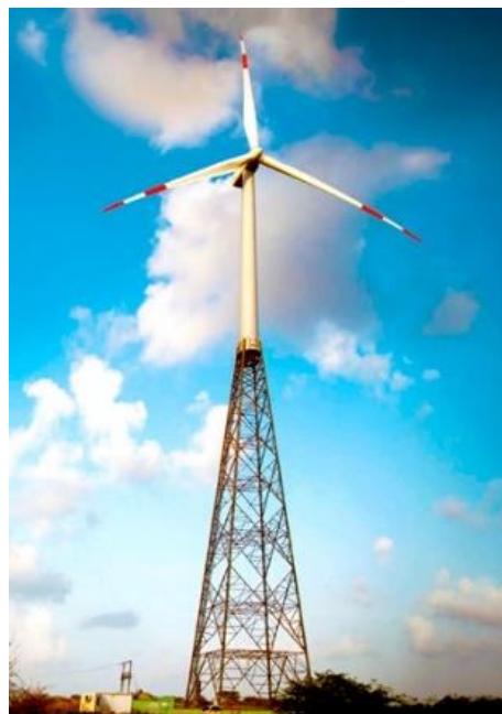
Figure 2.9: Suzlon Energy 120m hybrid lattice-steel tower ( www.suzlon.com )
