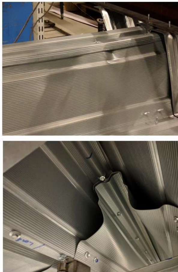
Figure 3.13 Local Web Buckling of LHP200, t=0.85\text{mm}
