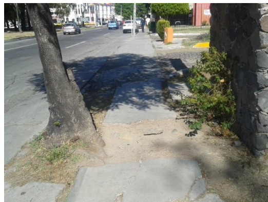
Figure 54: Unevenness caused by the tree in the sidewalk
