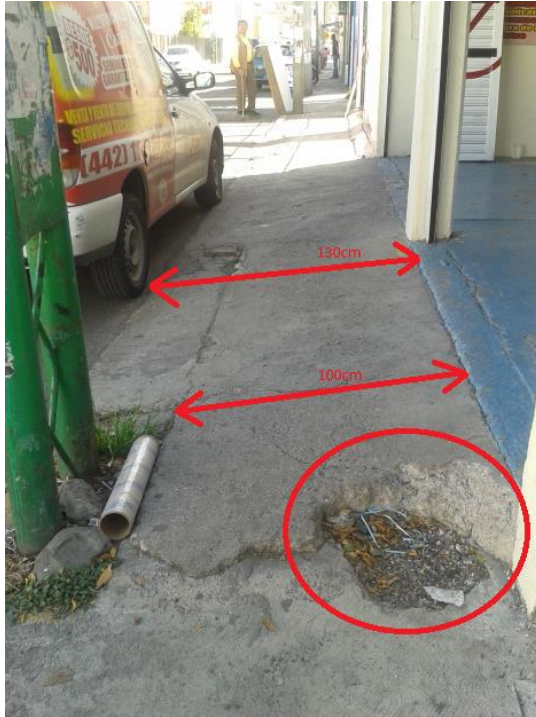
Figure 42: Hole on the main streets sidewalk and the longitudinal slope
