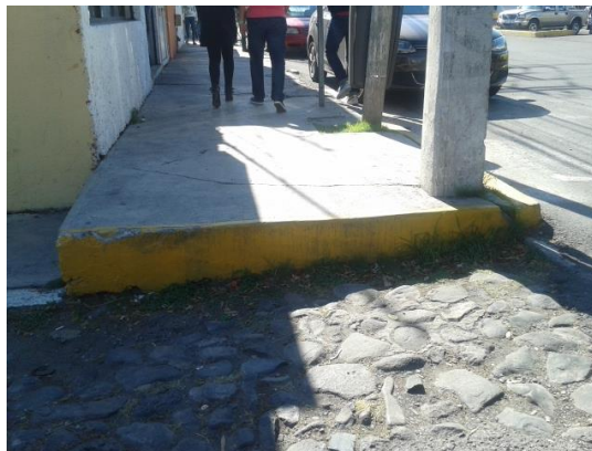
Figure 50: Very high step to the sidewalk
