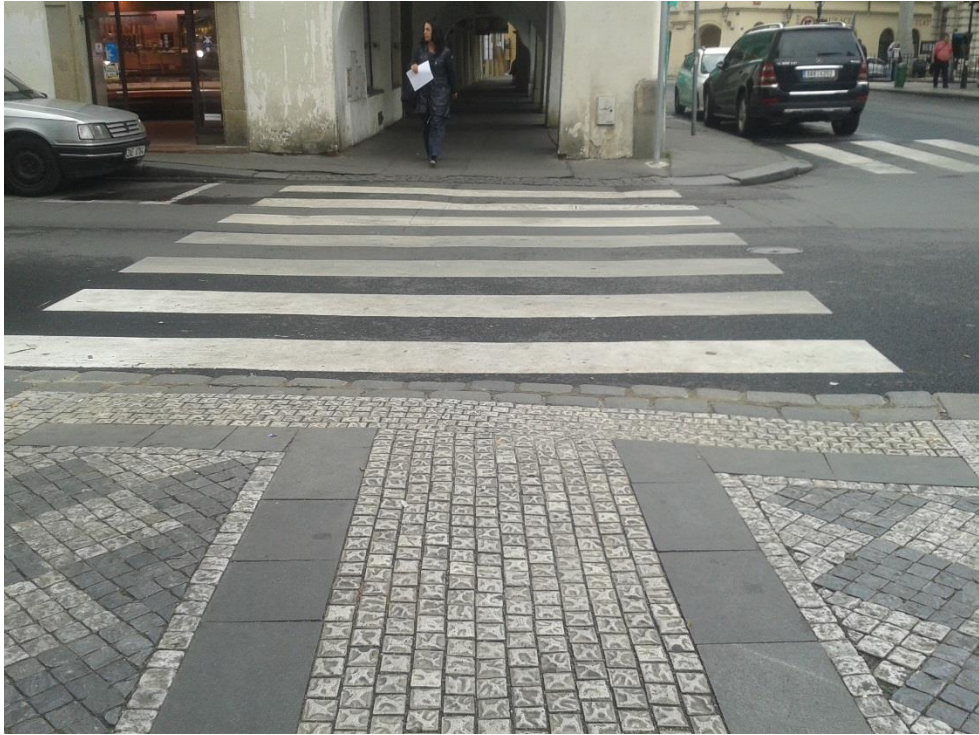
Figure 74: Missing tactile paving (on the other side of the street) and the guide line
