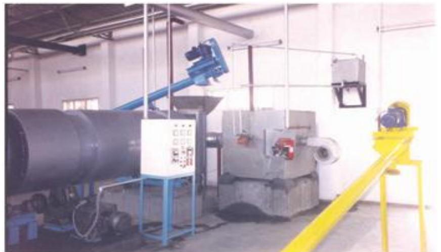
Figure 10. Rotary louver dryer
