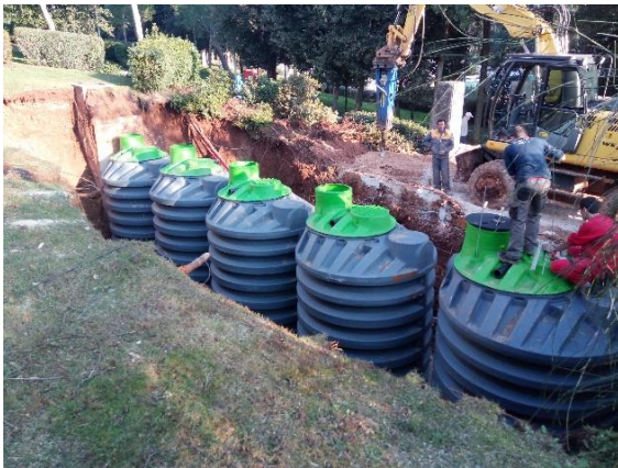
Picture 5: Installed tanks in a row
