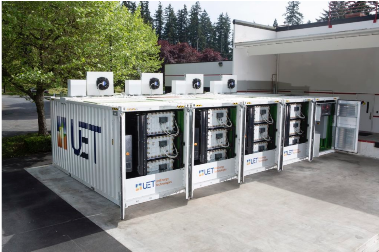
Figure 17 Flow battery energy storage (18)
