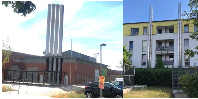
Figure A2.12 The Combined Heat and Power (CHP) Plants – standalone structure (left), included in apartment building basement (right) (source: Bardhyl Rama)
