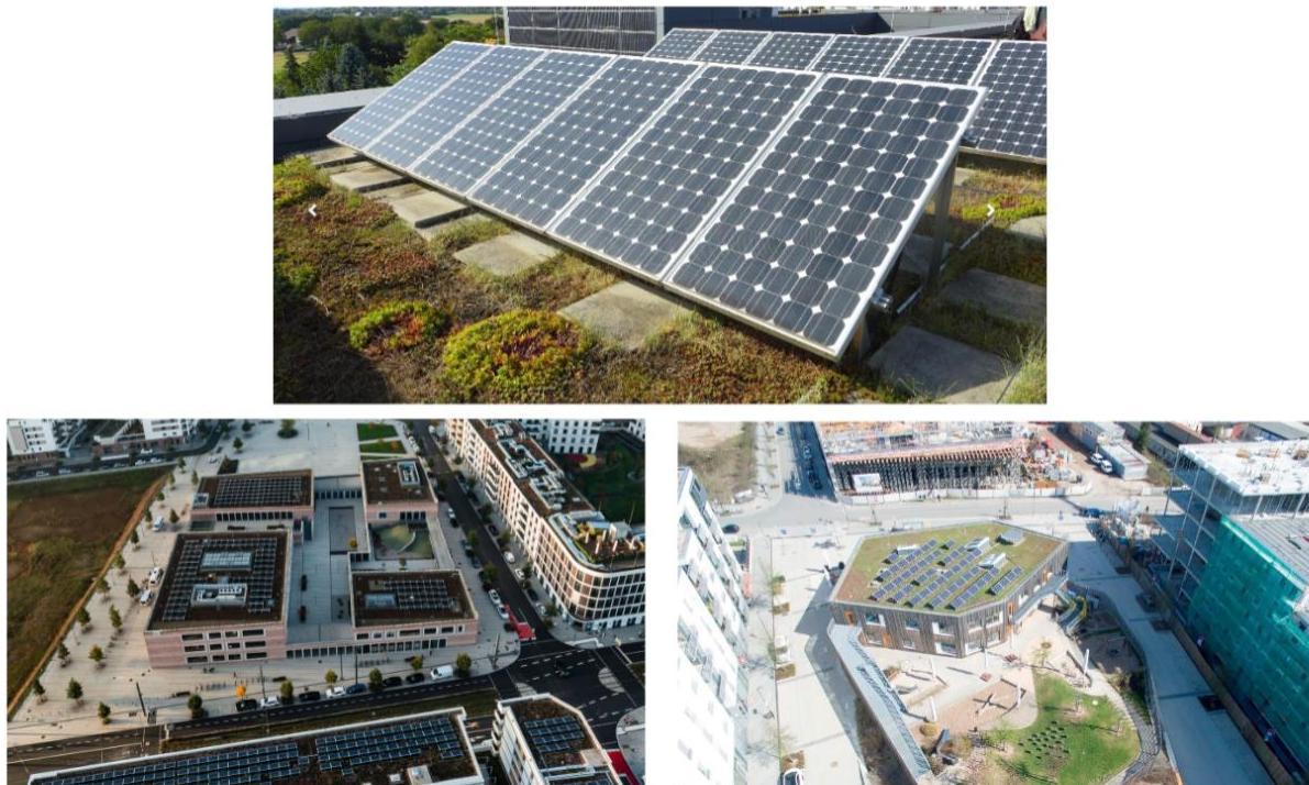
Figure A3.9 Photovoltaic solar panels arrays (source: city of Heidelberg (top), Frey Architekten (bottom))
