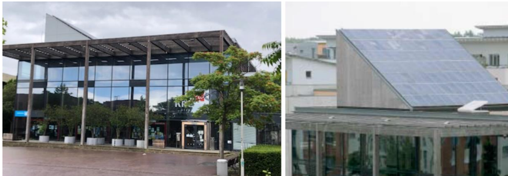
Figure A2.11 Photovoltaic installation at KroKuS (source: Bardhyl Rama (left), (Rumming K. et al, 2004b) (right) )
