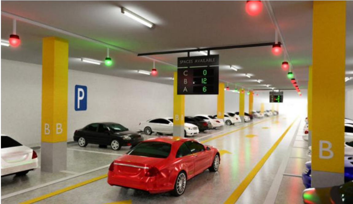
Figure 3.2: Parking technology - occupancy sensor lights. (Phasura 2022)
