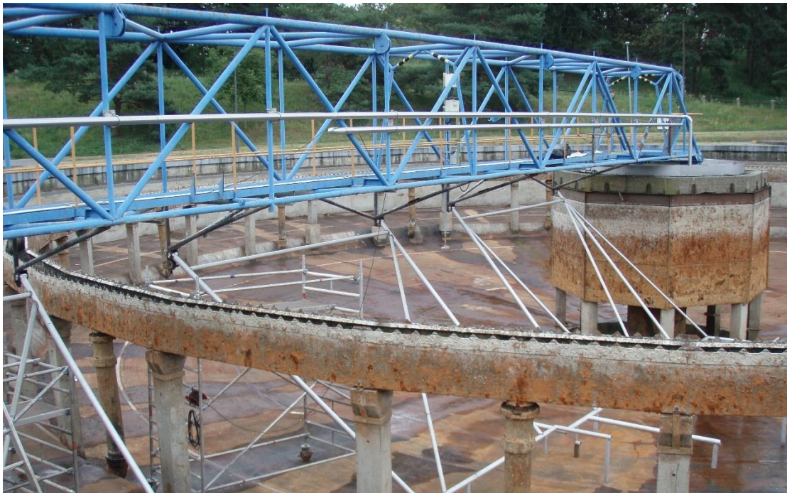
Figure 12 – Secondary settling tank at the CWWTP in Prague
