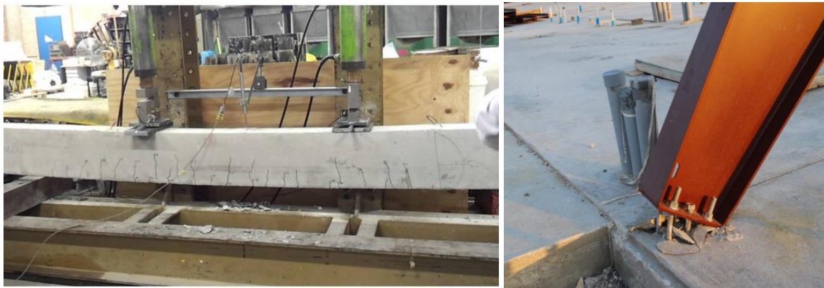
Fig. 16: Example of ULS exceeding for girders (left) and anchors (right)
