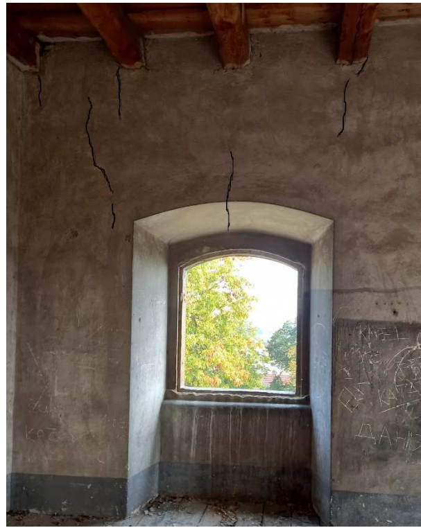
Obr. 3.36 – Shluk trhlin CV4.14
