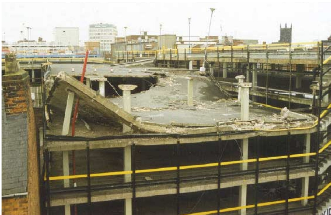
Figure 1.1 Collapsed top floor of slab at Pipers Row Car Park (Jonathan , 1997)
