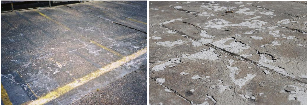
Figure 2.23 Typical examples of frost damaged slab
